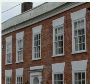
Camber flat arched render lintel above windows on the Horsford Hall facade
